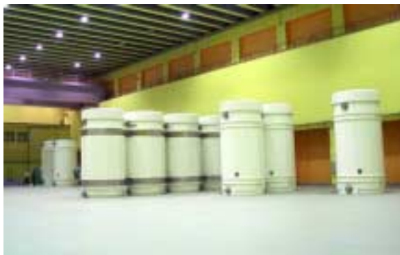
Centralised dry store for casks of HLW, the Zwiilag facility, Würenlingen, Switzerland
